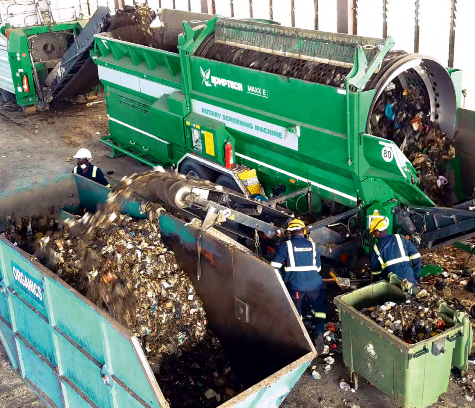
▲ Integrated Recycling And Compost Plant (IRECOP) – Location: Accra, GHANA Start of operation: 2019 Capacity: 200 tons per day
